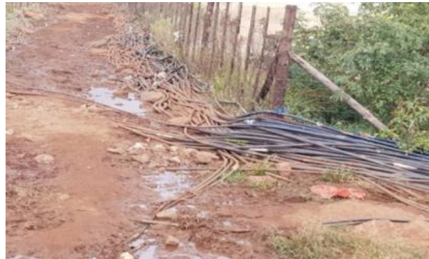
Illegal connections in Raliphaswa village Nzhelele
