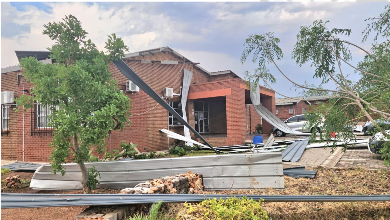
The roofing of the Municipal Traffic Offices was uprooted by the storm and heavy rainfall, leaving employees without office space
