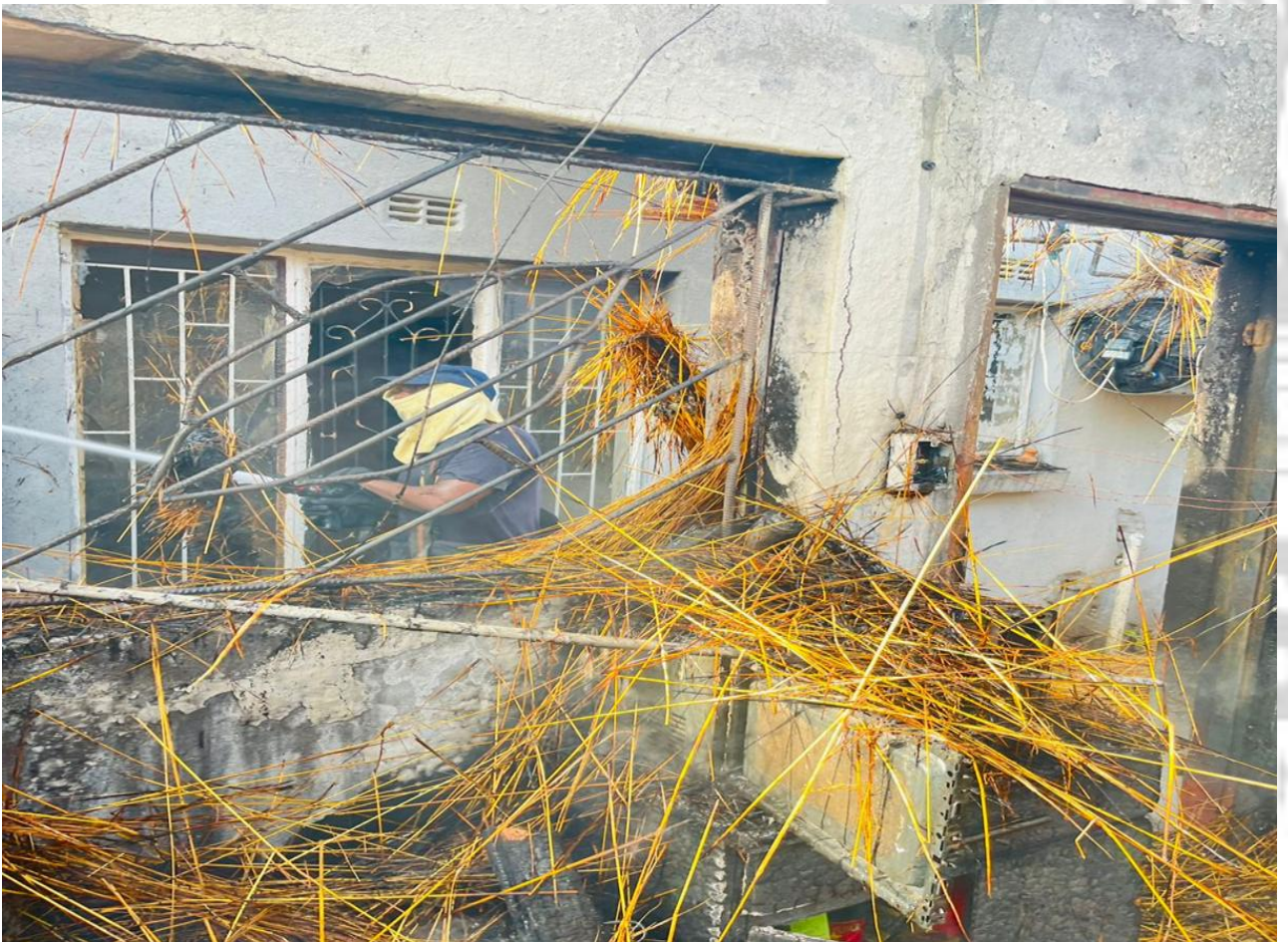
An incident of a house fire occurred in Longhomes, Ward 03
