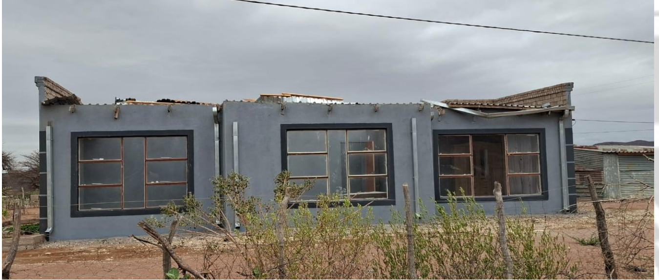
A household in Muswodi Tshisimani, Ward 07 was left without shelter after strong winds uprooted its roofing
